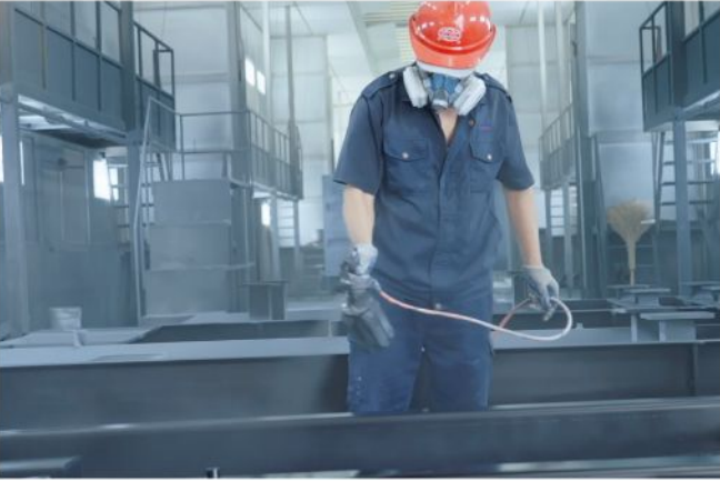
喷砂房 Sandblasting room
