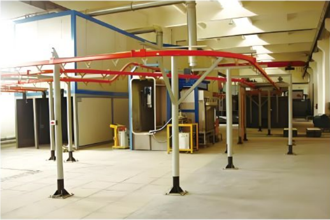
涂装生产线 Coating production line
